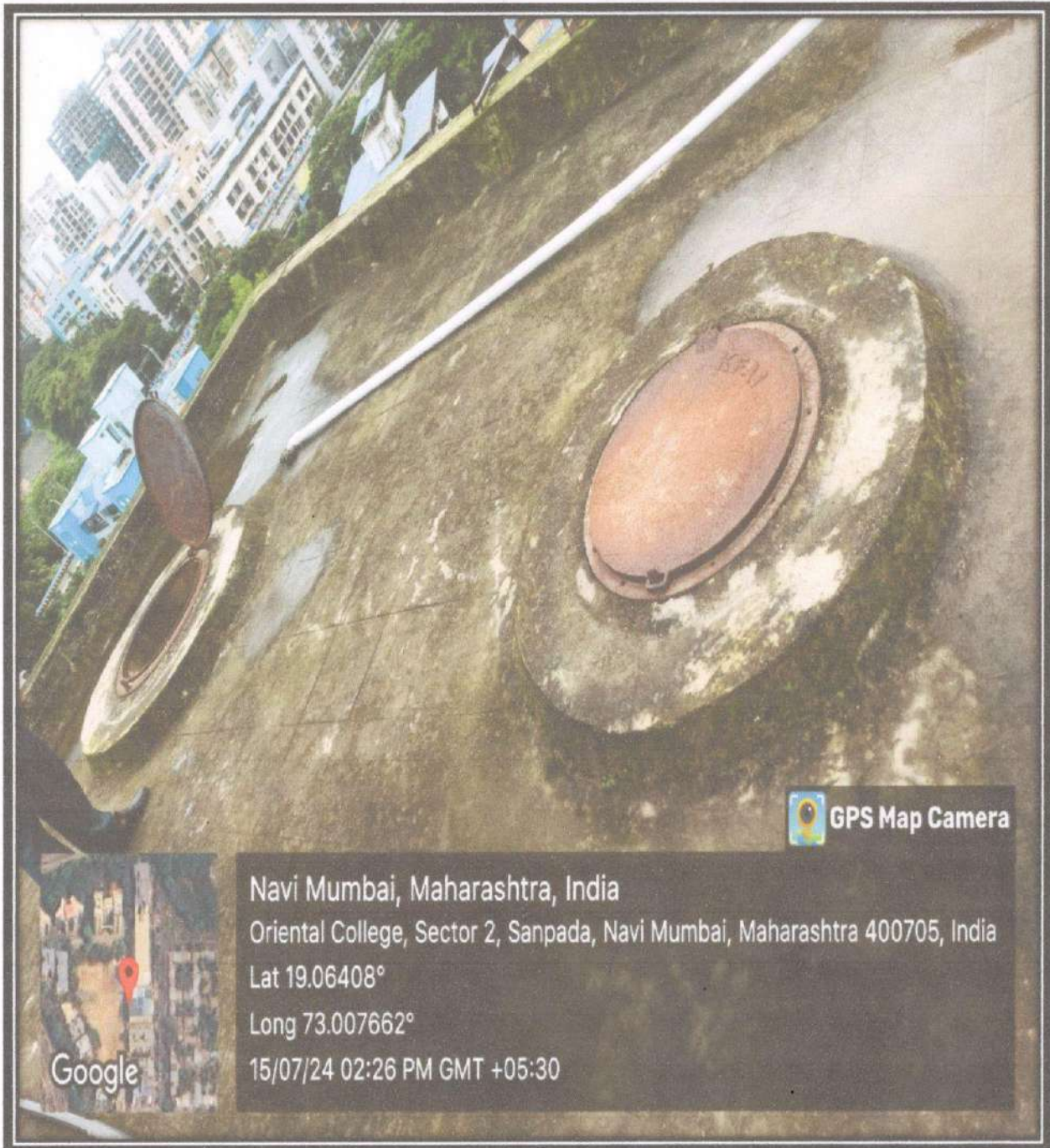
Photo: Over Head Tank in the campus building
